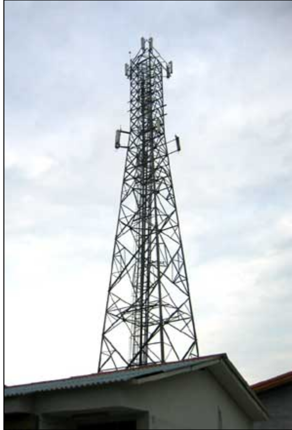
The airPoint Nexus PRO TOTAL was installed at the top of a 115 ft (35 m) tower at Nokandeh
